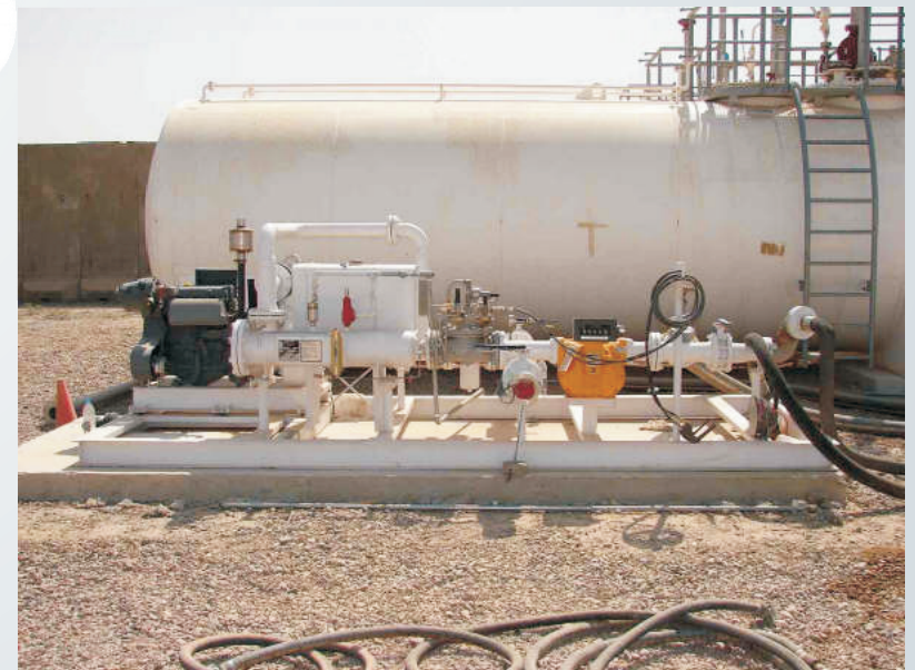
300 USGPM Diesel Driven Avgas Pump Skid US Air Force, Iraq
